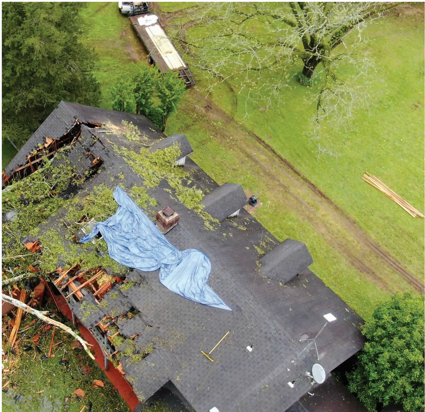
(Drone photo of damage in Hinds County)
